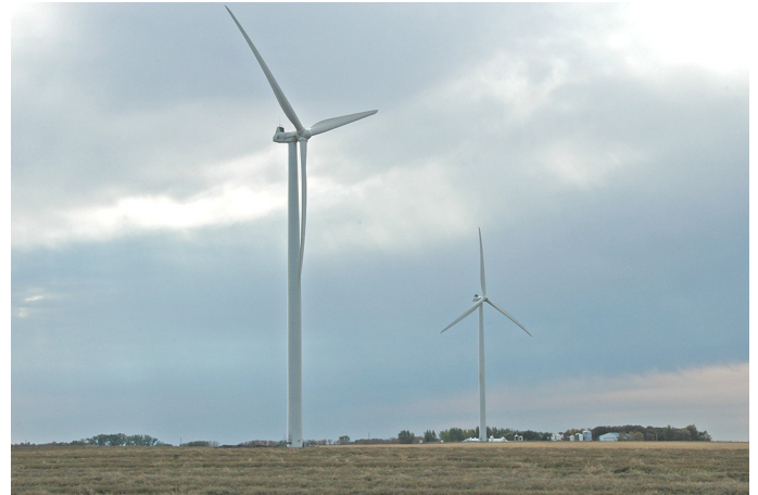
Figure 16 Turbines at Pattern Energy Group's St. Joseph Wind Farm Photography: Weldon Hiebert
